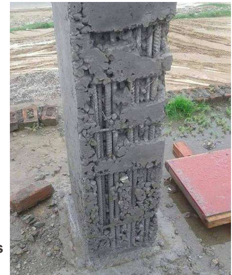
Placing issues (honeycomb)
